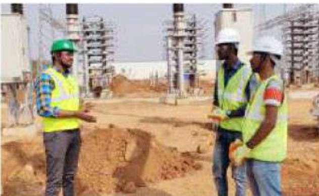
±800KV HVDC PGCIL RAIGARH - FILTER YARD ZONE2
