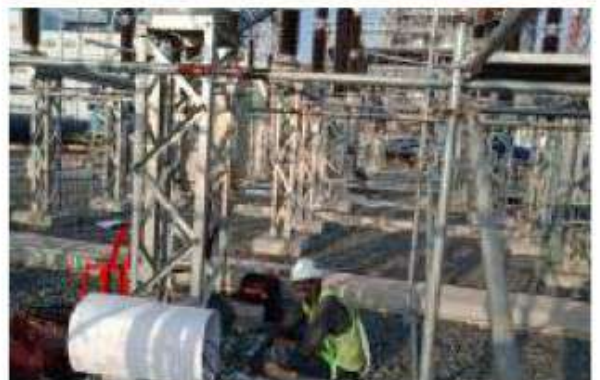
230kV Substation at CEL II Cambodia Project
