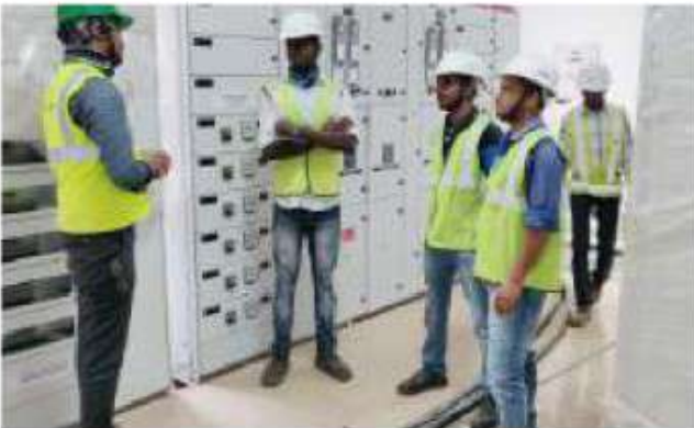
±800KV HVDC PGCIL RAIGARH - GIS ACDB
