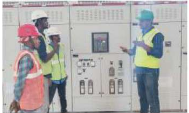
±800KV HVDC PGCIL RAIGARH - 415V ACDB POLE1
