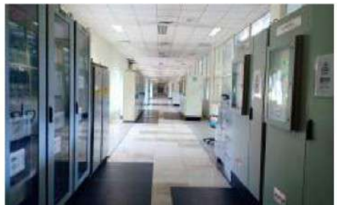
CRP Panels at Raigarh, 400kV GIS
