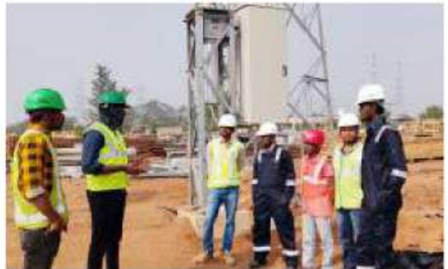
±800KV HVDC PGCIL RAIGARH - FILTER YARD ZONE1
