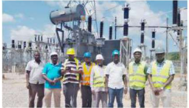
132/33kV Substation at 20MW Kabulasoke Solar Project
