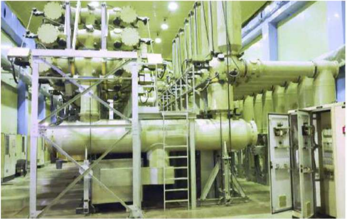
NHPC 240 MW Hydro Electric Power Plant
