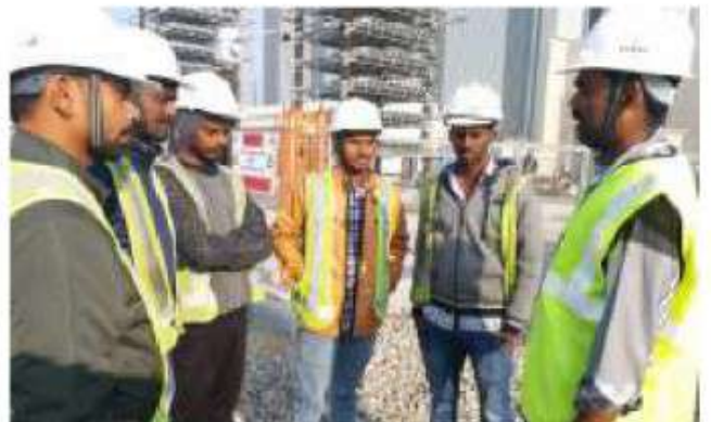
DC yard, \pm 800\text{KV} HVDC KURUKSHETRA
