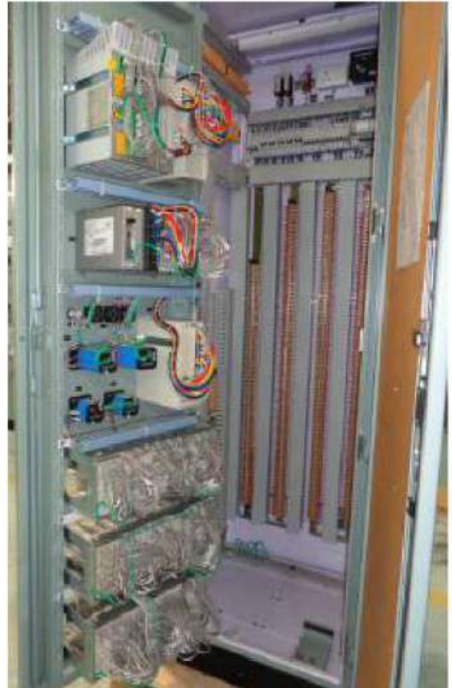
132kV Line Control and Relay Panel
