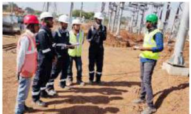
±800KV HVDC PGCIL RAIGARH - FILTER YARD ZONE2
